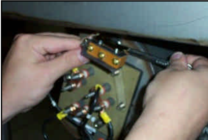
Tightening the brass fitting.
